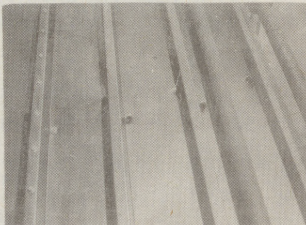
Fig.6. Sheetting tearing out (only at sheet/purlin fasteners)
